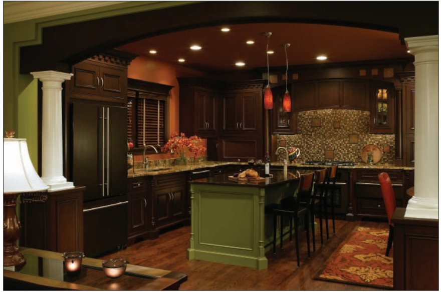
With advanced whole-home lighting control systems, residences can become more energy efficient and offer a greater level of convenience through features such as preset lighting scenes for each room.
