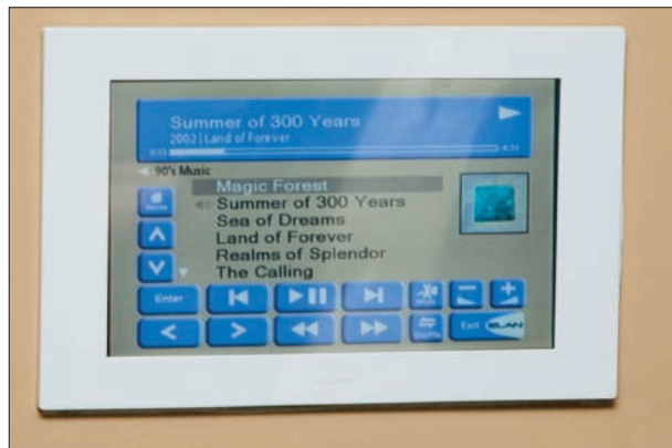
The centrally located touchscreens control the global lighting scenes for the entire property, the surveillance cameras, and the multiroom audio.
